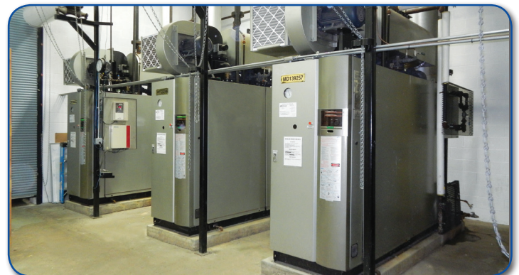
Three Miura LX-200 steam boilers provide efficient operation at Up to Date Laundry.
